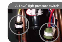
Low pressure switch High pressure switch
